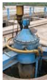
Hydraulic pump (Water is pumped up by hydraulic power.)
